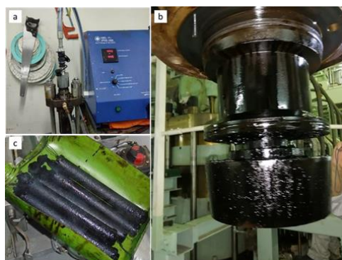
Figure 3. a. Fuel injector seizure, b. Fuel Pump Plunger and Barrel are sticky and unable to move, c. Damaged filter cartridge.
