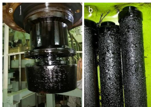
Figure 1. a. Fuel Pump Plunger and Barrel are stuck and unable to move, b. Damaged filter cartridge
